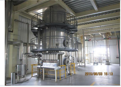
Deodorization tower designed for efficient odor removal and vacuum-based processing.
