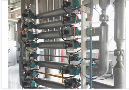
Bleaching section equipment for pigment removal and precision filtration.
