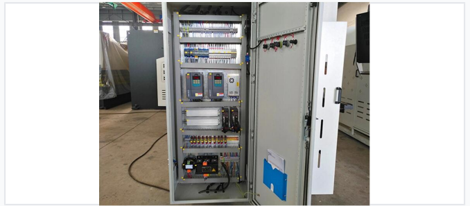
Integrated electrical control cabinet for system management.
