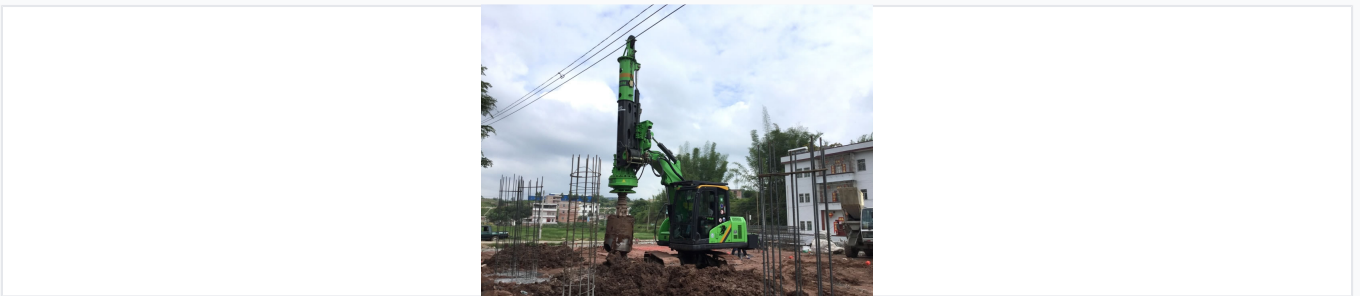
The rig is equipped with a versatile drilling attachment for precise pile foundation creation.
