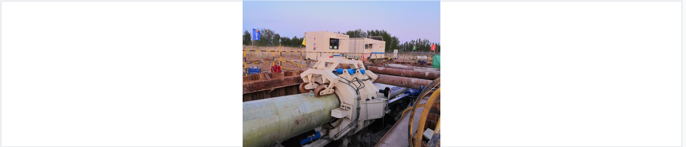
Operational setup showing the pipe handling and thrusting mechanism at a construction site.
