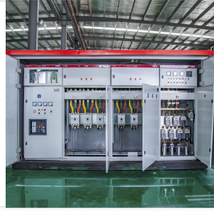
Integrated switchgear layout showing high-voltage and low-voltage compartments.
