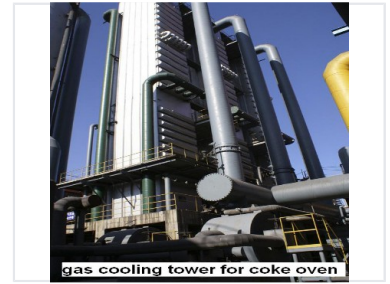
gas cooling tower for coke oven
