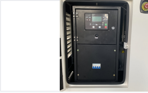
Integrated ComAp control panel with digital display and emergency stop safety feature.
